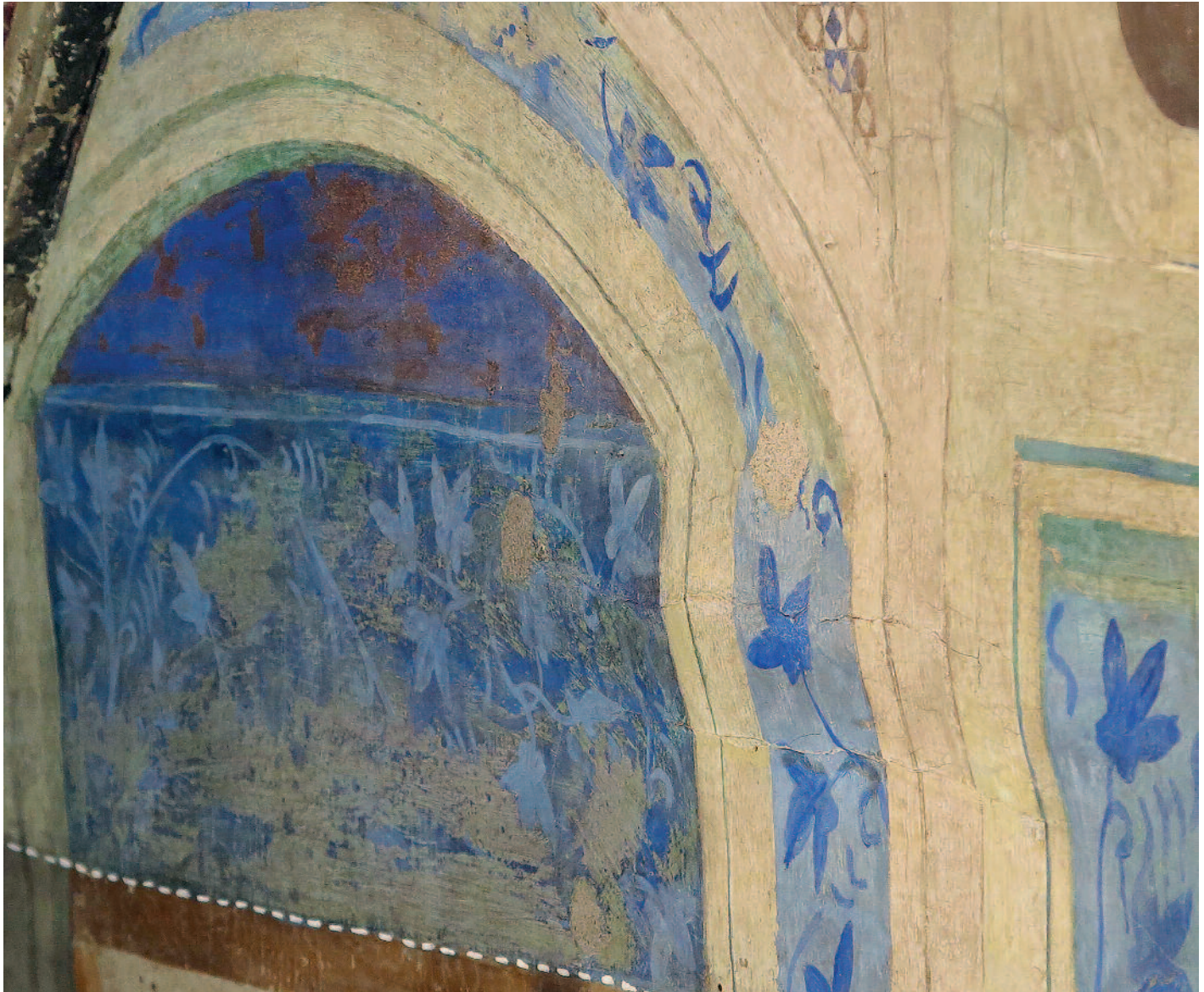
Convex deformation of painted plaster layer, Chapel of Saint-Martial, Palais des Papes, Avignon (France), 14th century; Photo: 2013, CICRP (Jean-Marc Vallet)
