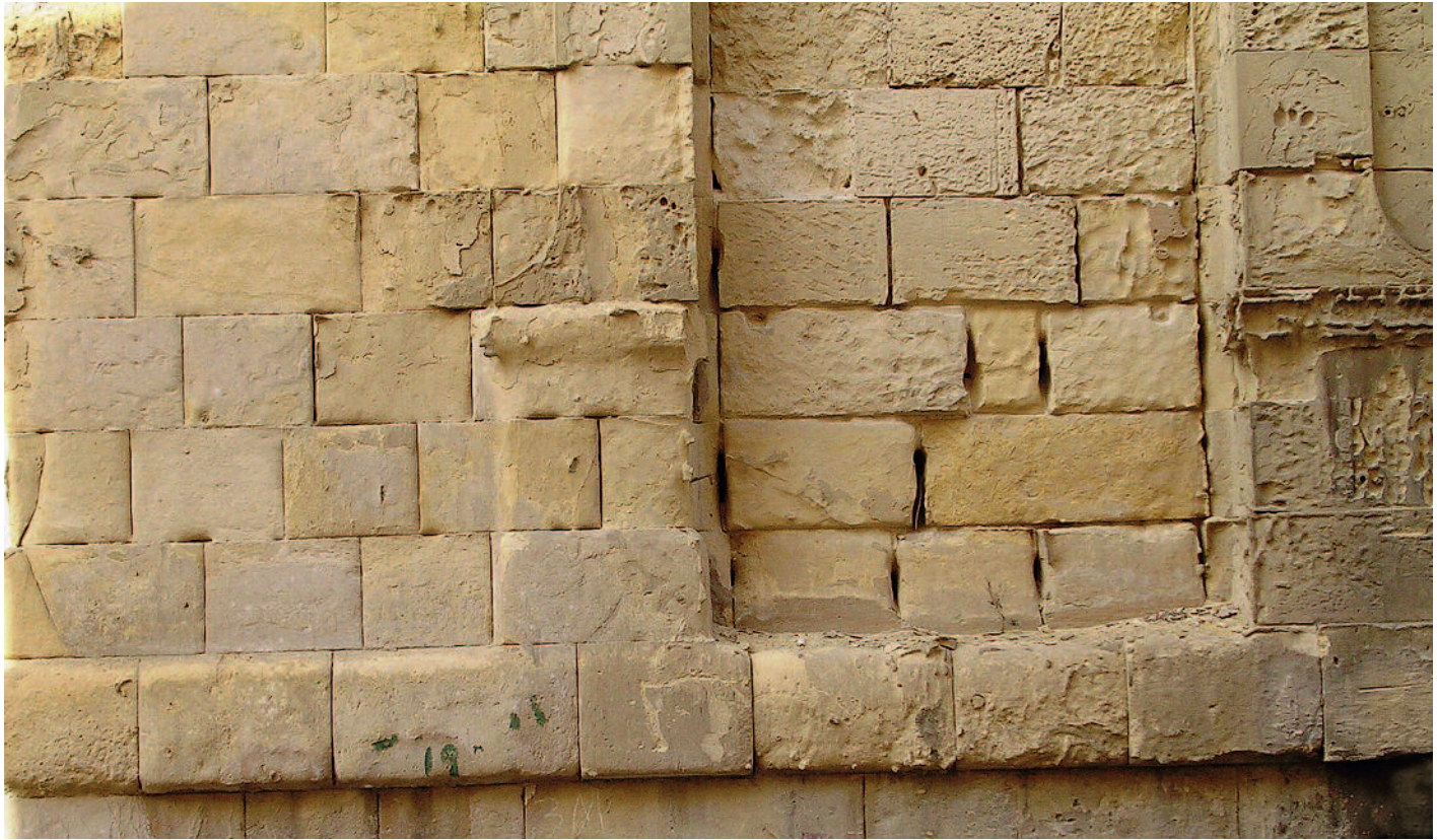
Wet-dry cycles, in the presence of soluble salts, lead to severe deterioration in porous limestone (Malta); Photo: 2008, UM (JoAnn Cassar)
