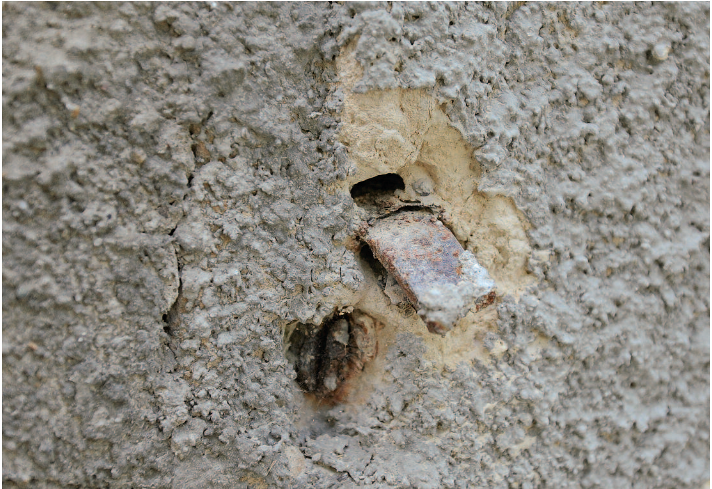
Corroded metal, building façade, Cluj-Napoca (Romania), 20th century; Photo: 2015, UAD (Adrian Rauca)
