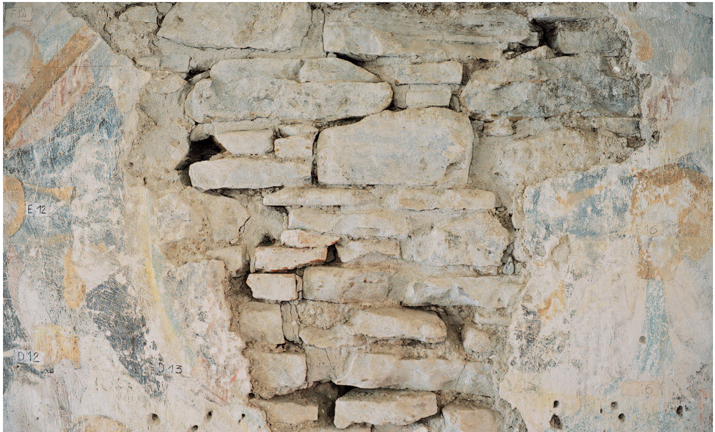
Loss of plaster shows masonry support (detail), Fortified Church in Apold (Romania), 13th century; Photo: 2014, UAD (Adrian Rauca)
