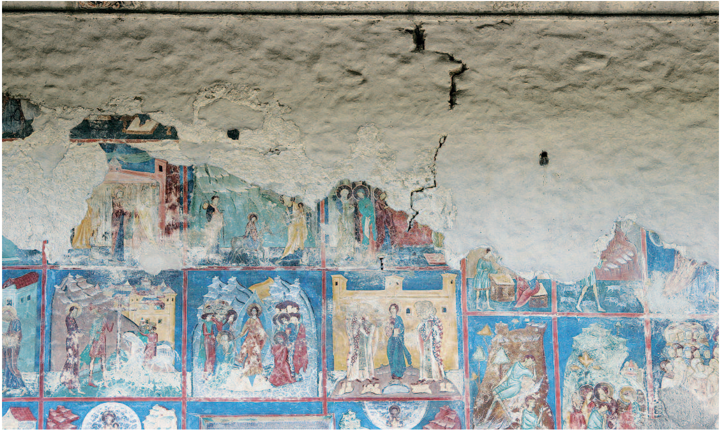
Crack caused by structural movement of a building, Arbore Church (Romania), 1502; Photo: 2012, UAD (Adrian Rauca)
