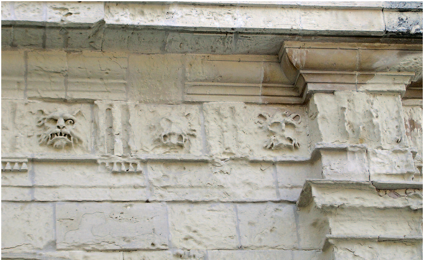
Fluctuating environmental conditions, especially humidity, have led to the deterioration of this salt-laden limestone (part of upper frieze in Globigerina Limestone), Greek's Gate, Mdina (Malta), early 18th century; Photo: 2008, UM (JoAnn Cassar)
