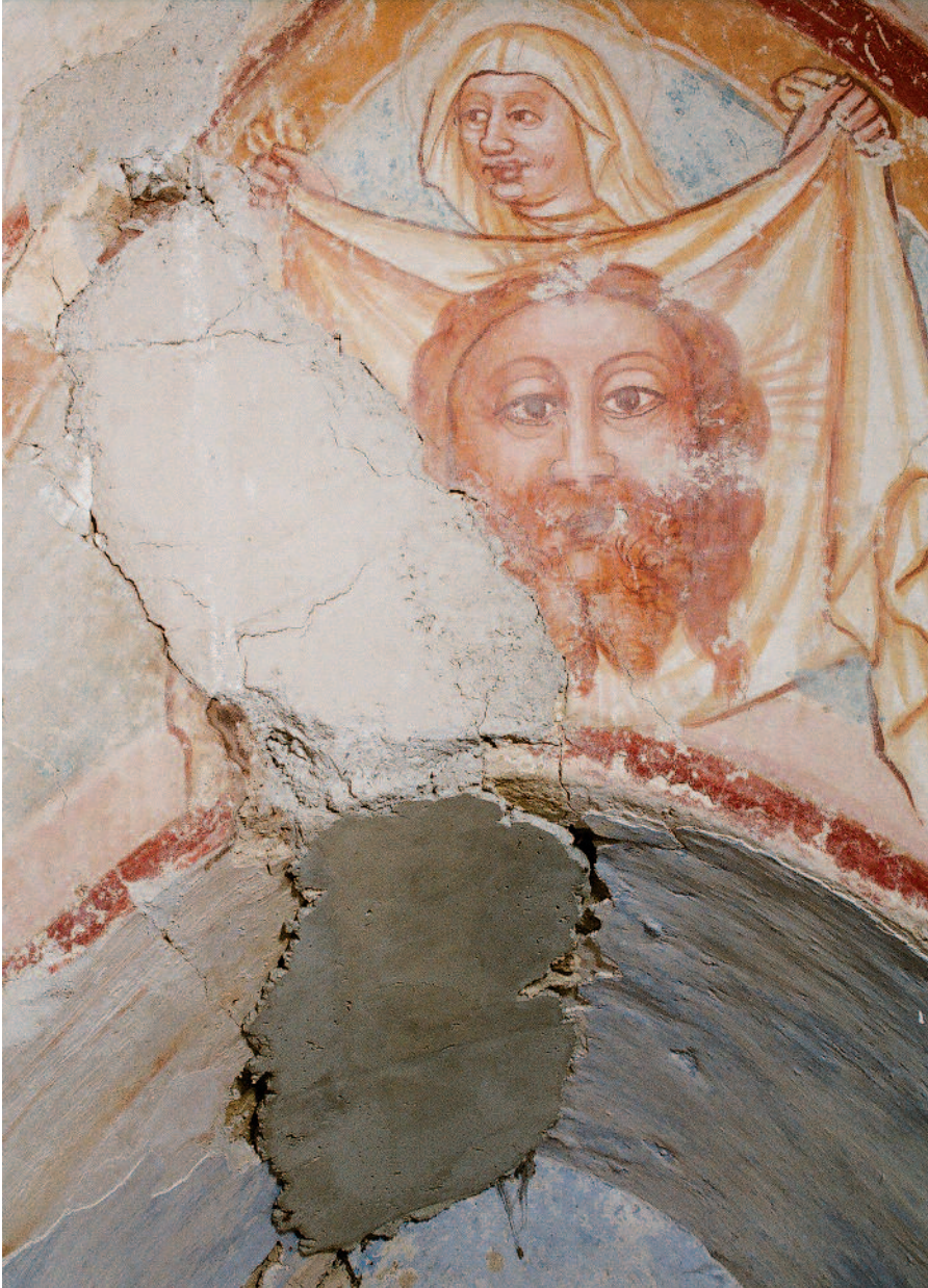
Incorrect plaster application, Chapel of St. John the Baptist, Ivanić Miljanski (Croatia), ca. 1450; Photo: 2002, HRZ (Ivan Srša)
