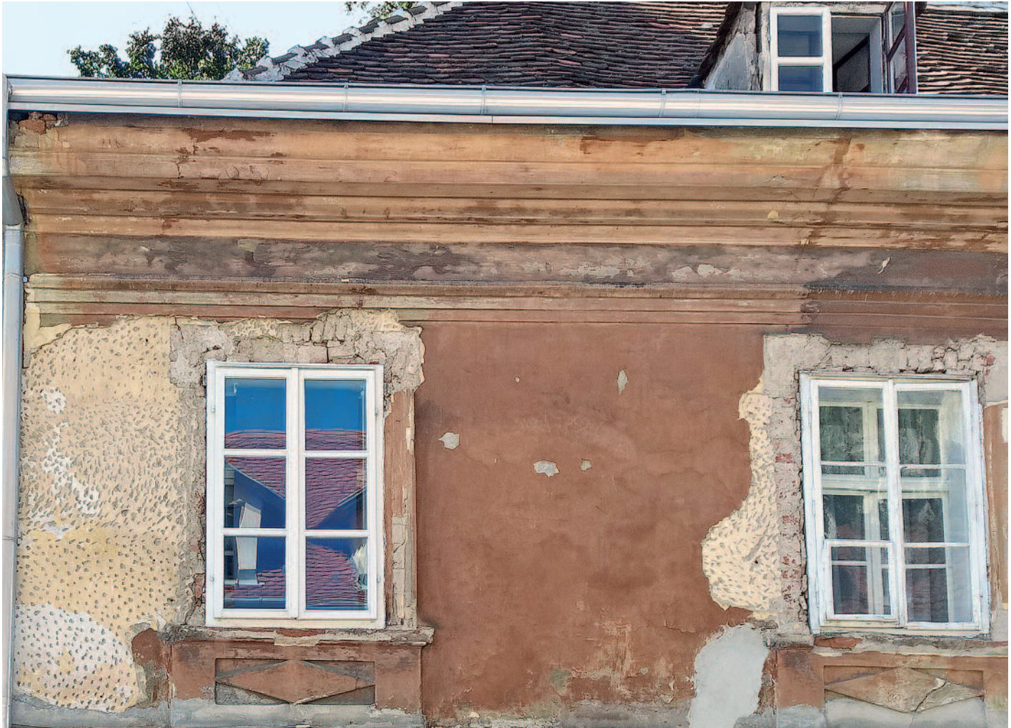
Losses of the top render layer allow a view of the layer beneath, showing traces of keying by hammering, historic building, Zagreb (Croatia); Photo: 2015, (Roland Lenz)
