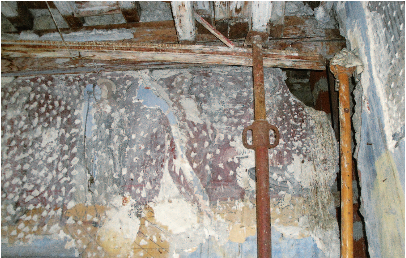
Collapse of overlying floor due to a structural fault, "Pantagruel" Building, Cavaillon (France), 15th century; Photo: 2011, CICRP (Jean-Marc Vallet)
