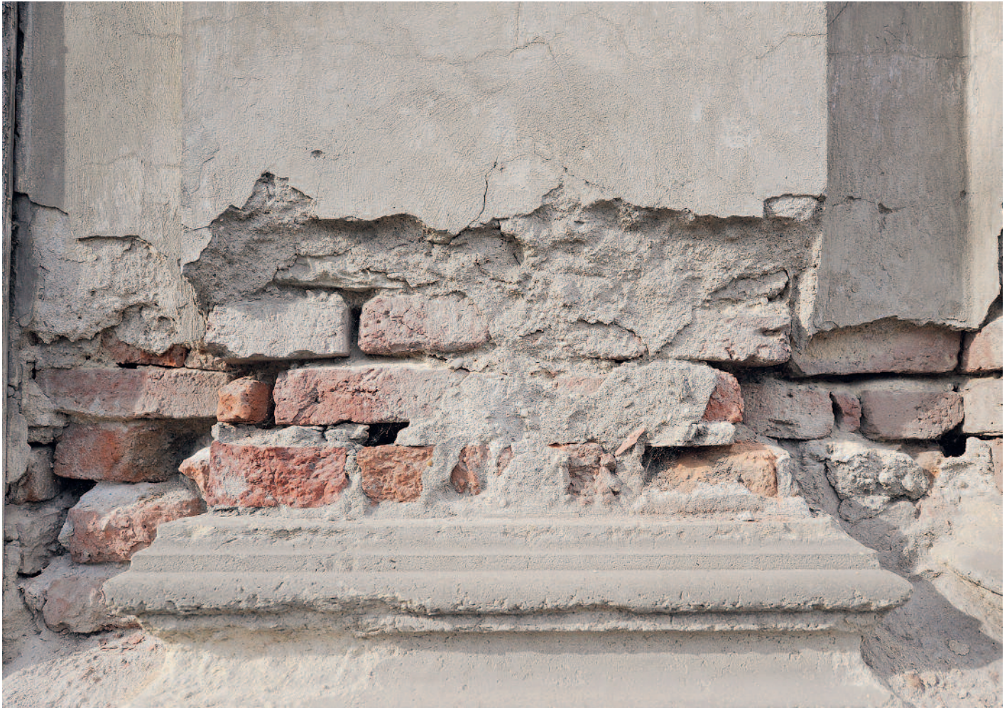
Crumbling building façade, Cluj-Napoca (Romania), 19th century; Photo: 2015, UAD (Adrian Rauca)
