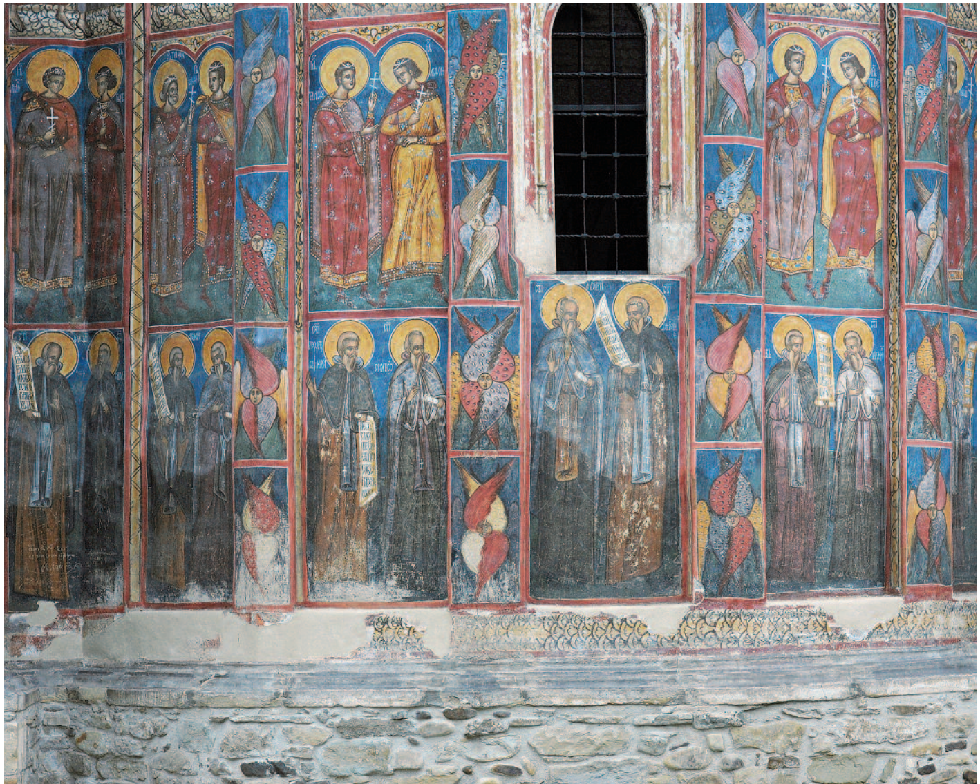
Rising damp visible as colour saturation, Moldovița Monastery (Romania), 1532; Photo: 2003, UAD (Theo-Sandu Mureșan)
