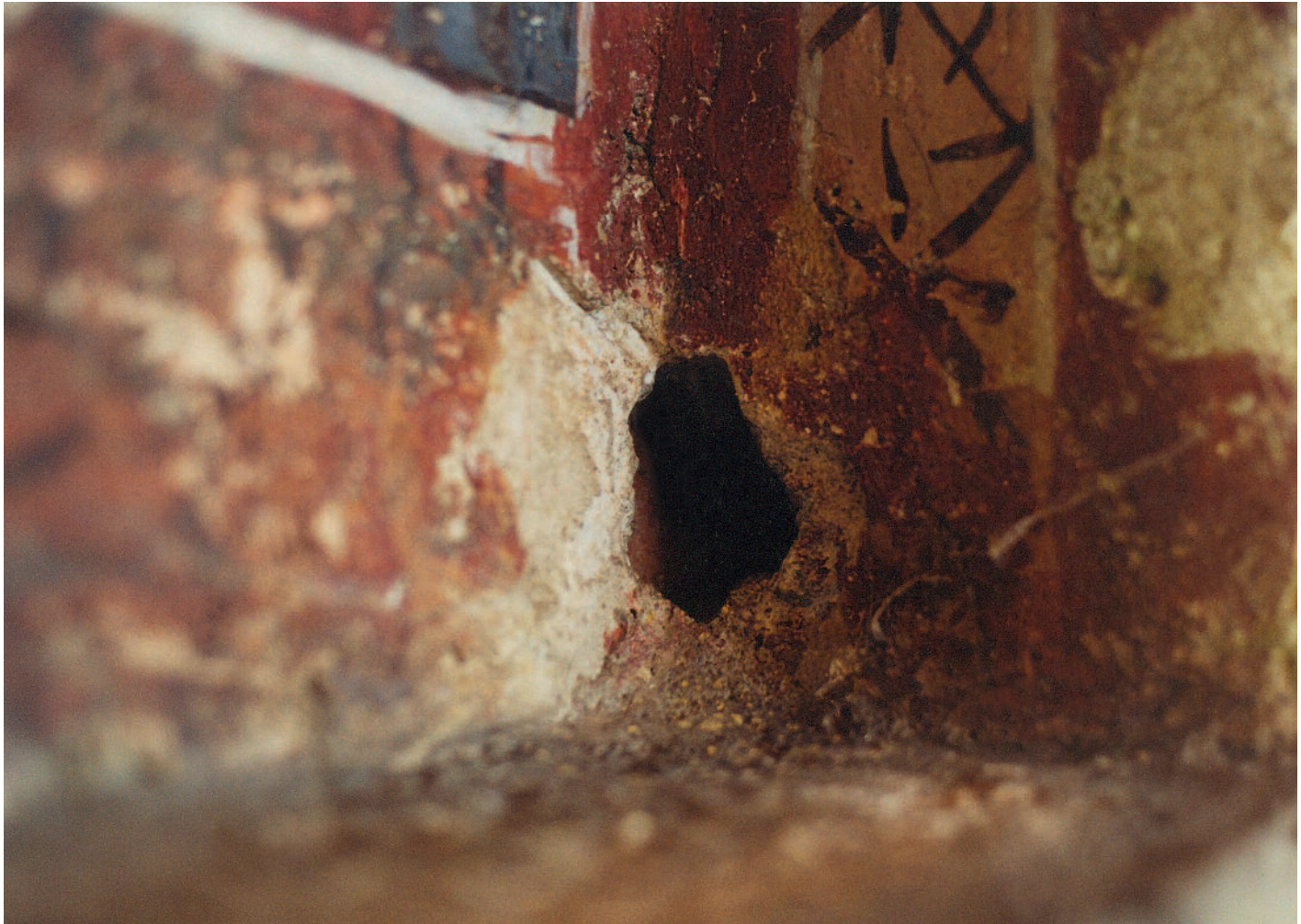
Deep hole in external wall painting, Moldovița Monastery (Romania), 1532; Photo: 1993, UAD (Theo-Sandu Mureșan)
