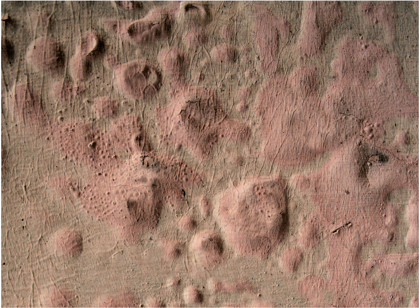
Paint layer showing bulges, Secco wall painting, Cluj-Napoca (Romania), 19th century; Photo: 2015, UAD (Adrian Rauca)
