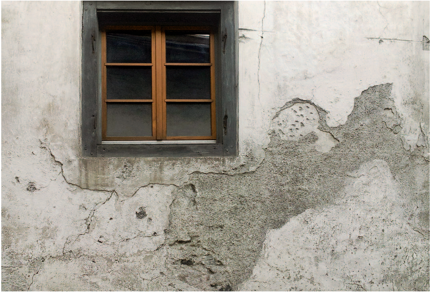
Plaster layers with final render above, historic building, Santa Maria Val Müstair (Switzerland); Photo: 2015, HAWK (Angela Weyer)
